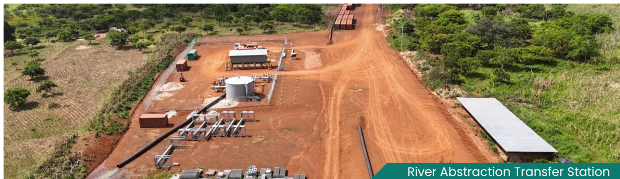
River Abstraction Booster Station
